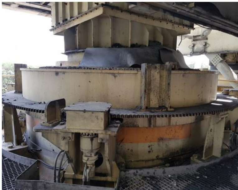
Figure 5.6. Metso MP2500 secondary crusher.
