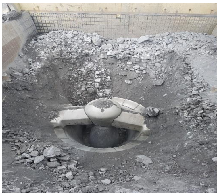
Figure 5.5. ThyssenKrupp KB63-89 gyratory crusher.
